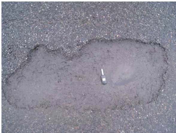
Figure 2 Observations recorded on test section 2 (central France specimen) (a) Rise of a head of water in a pothole in the PA layer (b) Borehole sample with disaggregated PA
