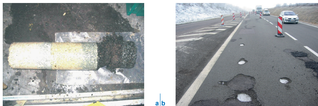
Figure 1 Pavement disorders in north-eastern France (a) Pavement structure borehole sample (b) Pattern of potholes tens of cm in size
